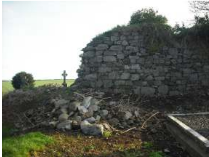
Vegetation removal & resultant collapse, Grallagh Church
